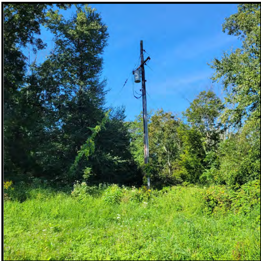
Phot 15: Pole-mounted transformer. Photo facing west.
