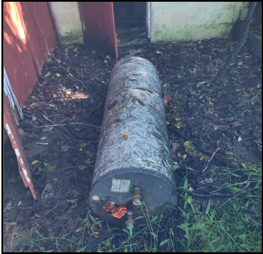
Photo 5: Hot water heater outside Building #1 utility room.
