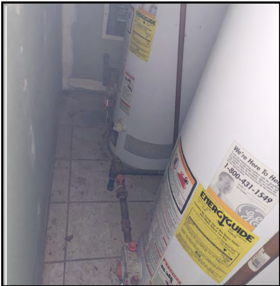
Photo 19: Hot water heaters in “Boiler Room” of Building #11.
