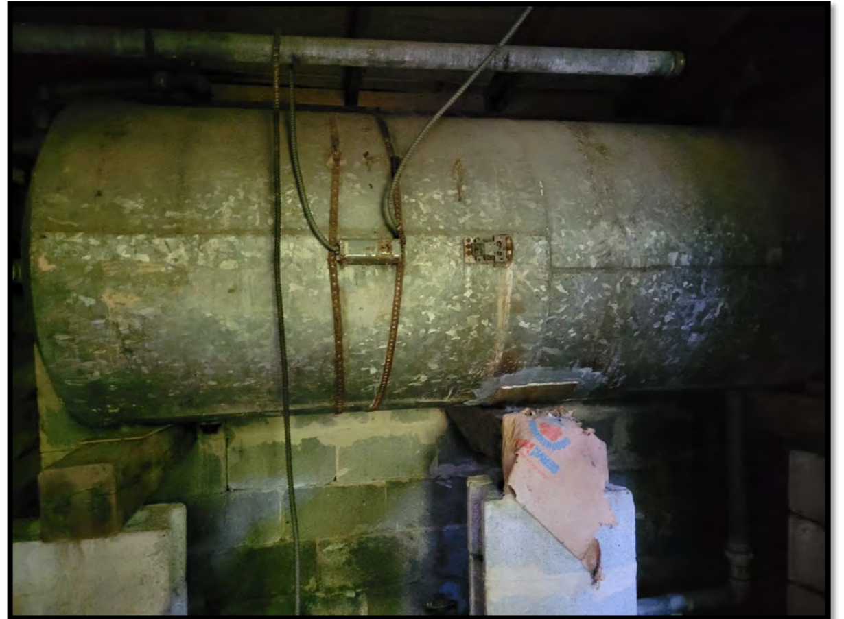
Photo 4: Presumed hot water holding tank in Building #1 utility room.
